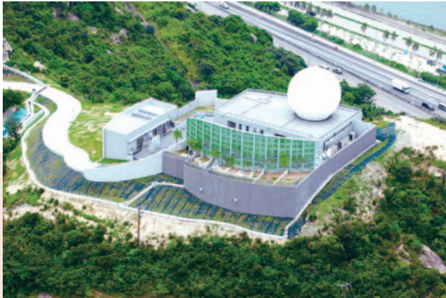
Construction of a station for a weather radar for the Architectural Services Department 為建築署建設天氣雷達站
